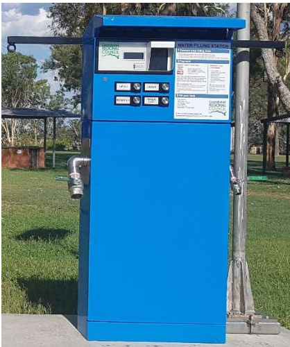
Inglewood Water Fill Station Location: Brook Street side of Lions Park, Inglewood
