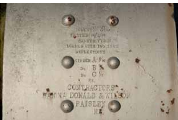
Figure 9 Construction detail of western girder. Made by Donald and Wilson, Paisley, Scotland
