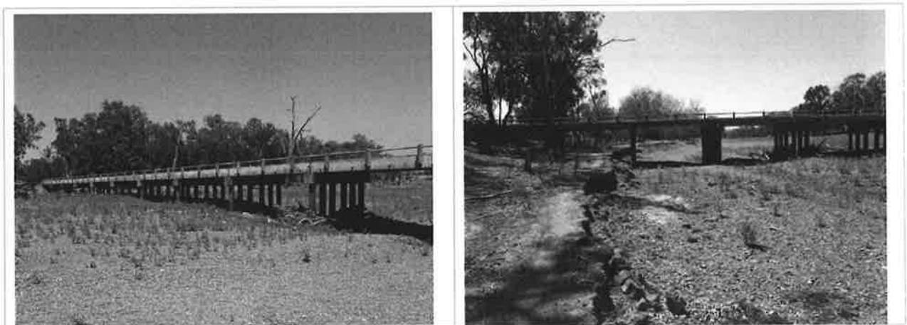
Figure 1 View of bridge from northern bank showing sediment build-up (L) and outer bank erosion (R)
